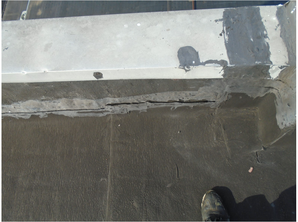
Photo P9 Close up of open base flashing.
