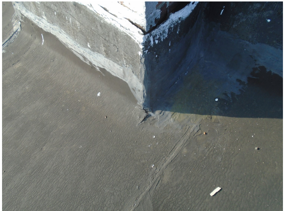
Photo P6 Open base flashing at chimney. Also cracked open hole in roof.
