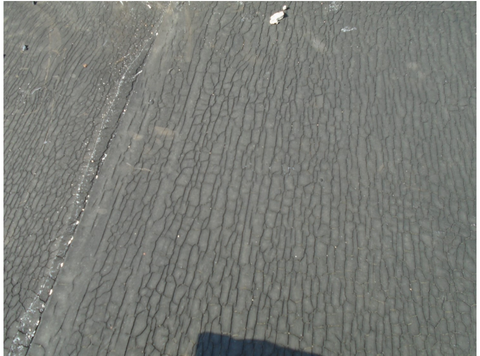
Photo P5 Typical cracked modified bitumen roof surface
