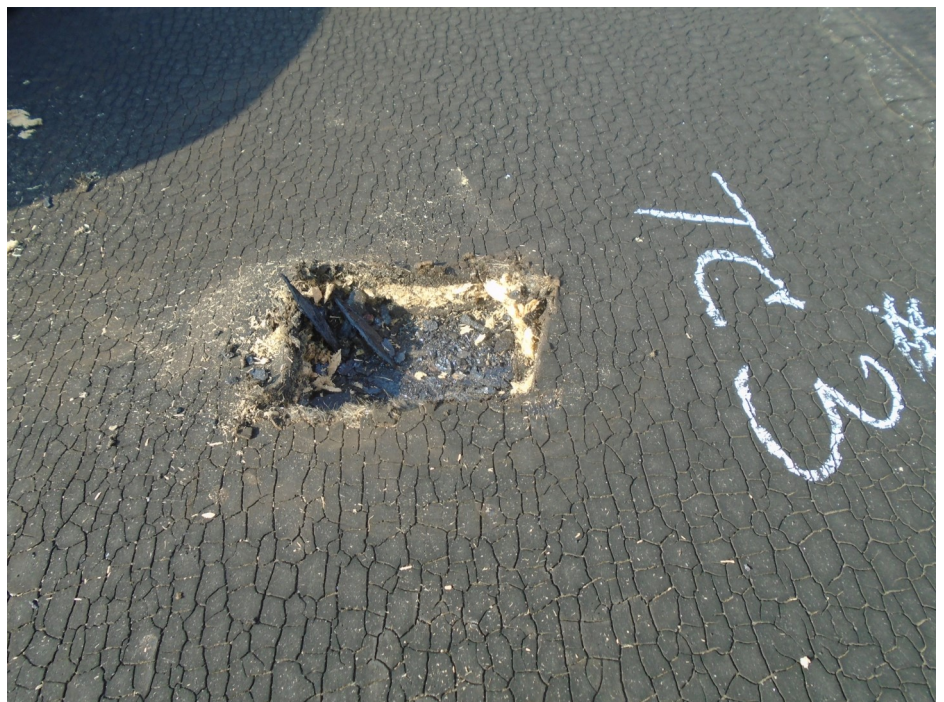
Photo 11 Photo of Test Cut #3. Note cracked and deteriorated roof.
