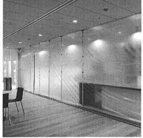
Protecting Sensitive Research Lab – When it is critical to keep dust contained, commercial remodeling companies often use ZipWall® barriers to seal off the worksite. This beautiful installation is in a scientific research building near Boston.
