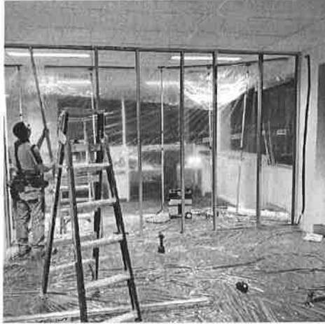
Commercial Job Made Easy by ZipWall® – One of the features contractors love most about ZipWall is how quick and easy it makes prepping the job site. Posted by OS Projects.
