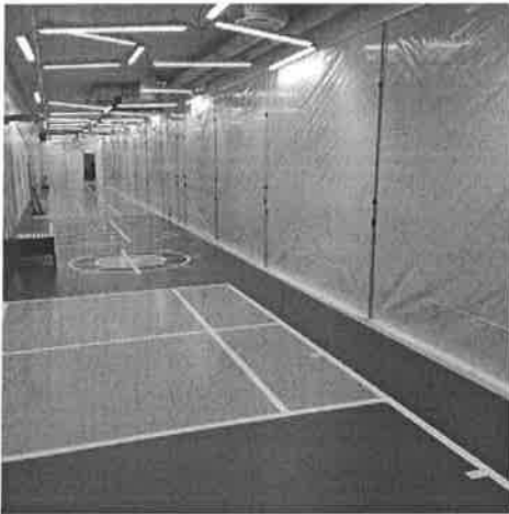
Dust Protection for Remodeling a Gym – This perfect ZipWall® barrier was set up to section off the work site and allow the gym to continue to operate during the remodel. Barrier set-up and image by Sellco, Netherlands.
